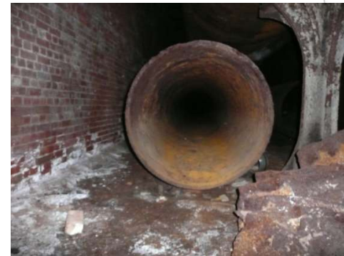
TYPICAL WROUGHT IRON PIPE AND CAST IRON PEDESTAL WITH SADDLE - MASONRY ATTIC
