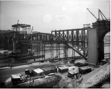
1927-02-20 High Bridge General View from Harlem River Drive Looking NE (Municipal Archives)
