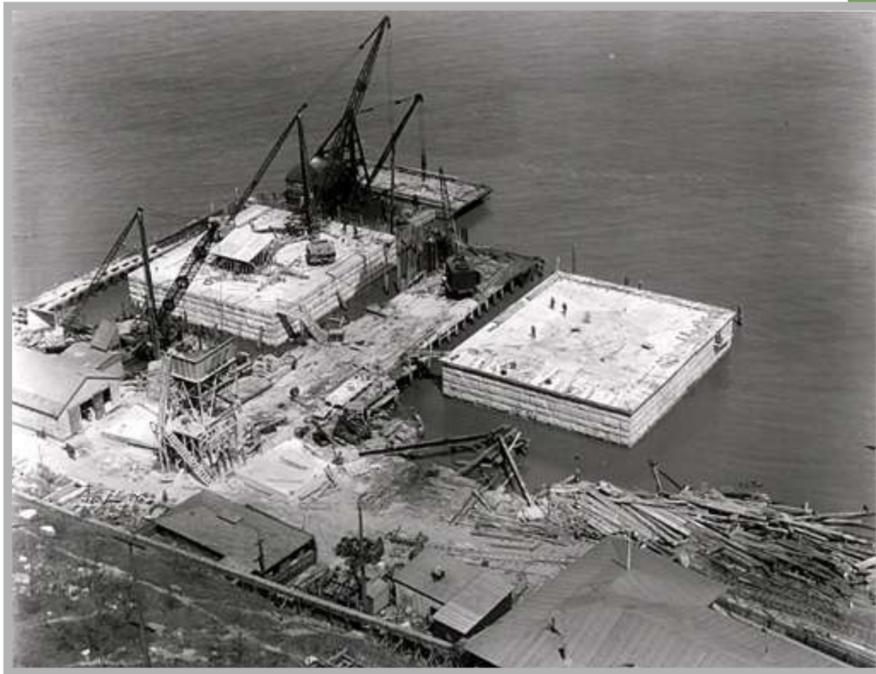
Cofferdam and Footing for New Jersey Tower Circa - May 1928 Center of Tower – 76 Feet from Shore
